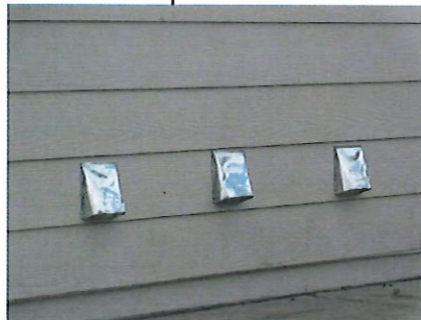
Nixon Townhome Wash House damage to vents
